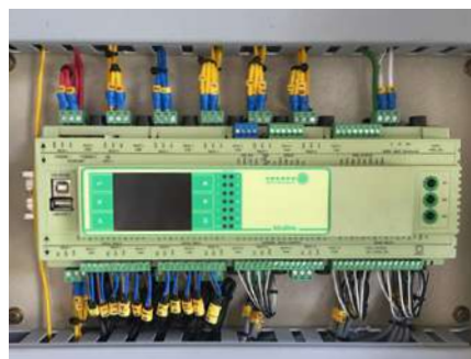
RDM's Intuitive TDB - HVAC and refrigeration controllers with PLC software built-in - manage and monitor all equipment.
